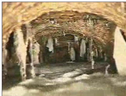
Zoom camera technology detects conditions that require further attention. Upper photo, grease buildup; lower photo, root intrusion, a source of infiltration and a potential cause of blockage.
